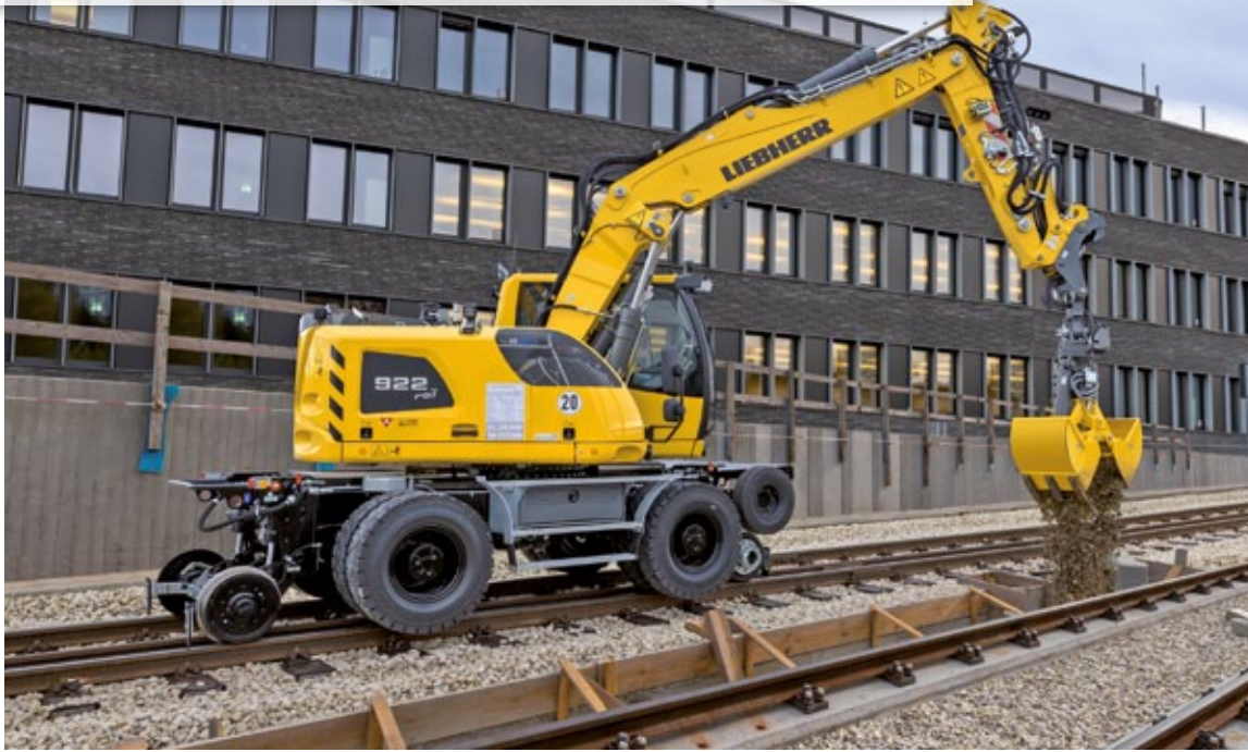
The 'A 922 Rail Litronic' road-rail excavator is used both in track construction and in classic earthmoving work.
