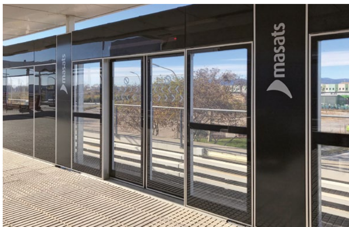
High platform screen doors in Barcelona
